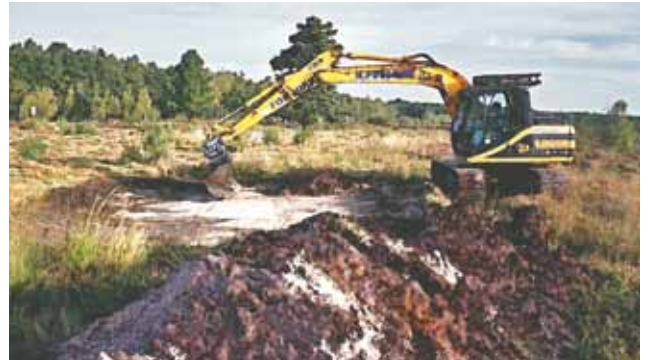
Machinery such as a 13 tonne, tracked, 360° excavator is suitable for creating natterjack scrapes (John Buckley)
