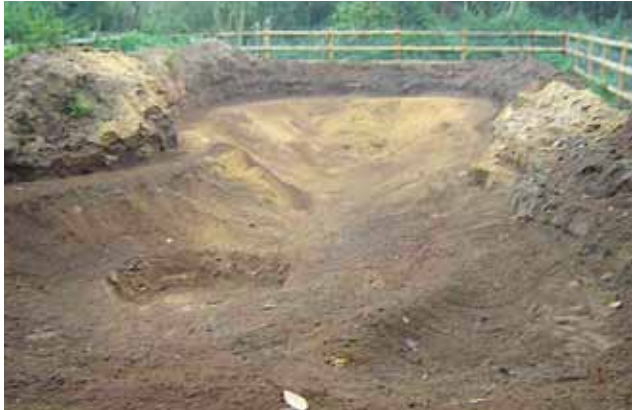
Here the butyl liner has been covered with a geotextile layer, topped with a 30 cm depth of sand from the excavation site (Duncan Sweeting)
