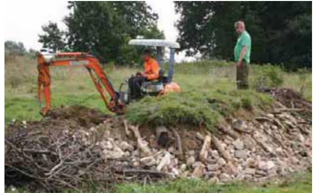
A reptile bank under construction. Turf has been stripped to create a shallow pit to receive a pile of hardcore and logs. This will be covered with the stripped turves (Lee Brady)
